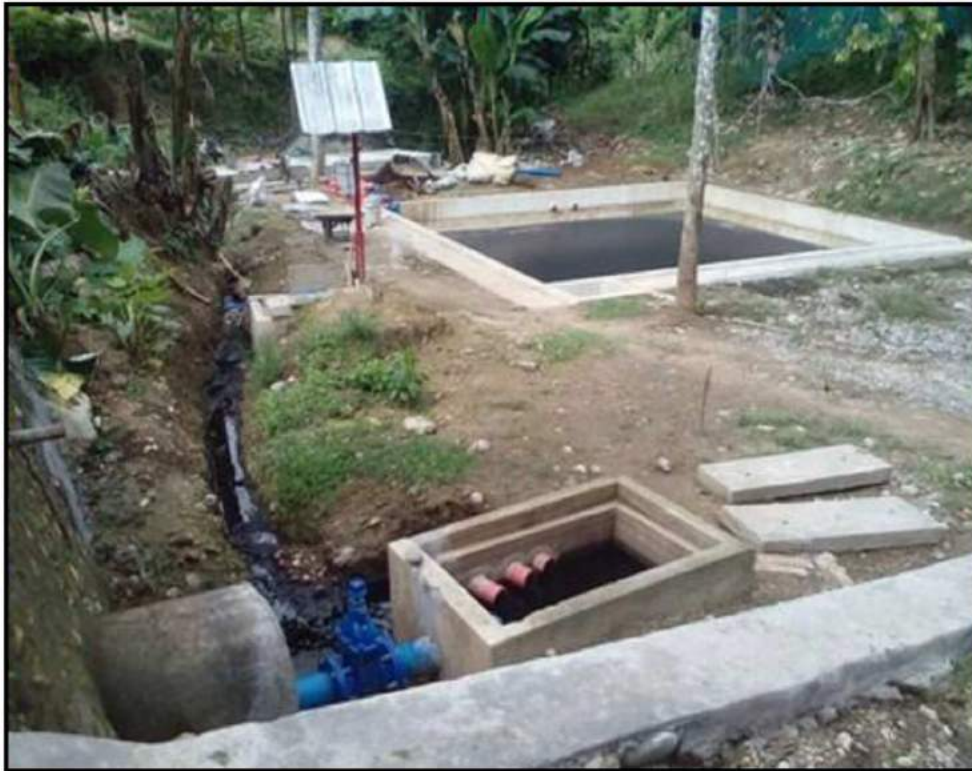
Figure 6. The leachate treatment facility of the dumpsite
